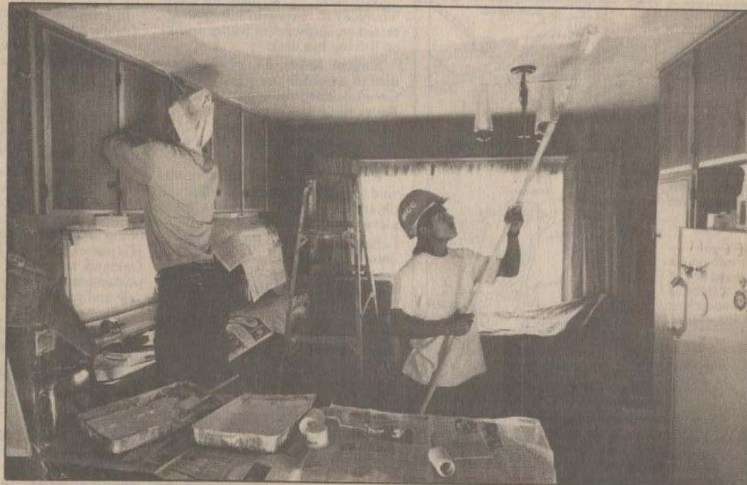
HELPING HANDS: Fernando Montenegro (left) and Gil-dardo Azueta paint the ceiling at Bunnye Wengren's mobile home in Novato. They are with the Marin Conservation Corps Elder Service Project.
