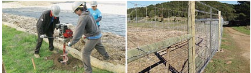
In January 2009, CCNB corpsmembers completed 1,800 feet of perimeter fencing around the project site to keep deer out.
